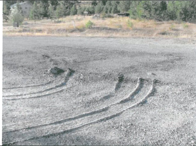
Damage caused by construction traffic. 9/9/08
