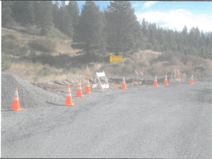
Even public works thinks it is "broken". This work was to prevent the snowplows from getting stuck again. 9/21/08
